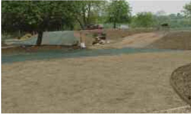
Newly landscaped installation... Green TurfProtecta™ laid and covered with a layer of topsoil and seed.
